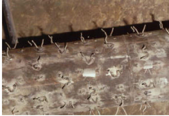
Refractory anchors used in waste incinerator operating between 1300-1700°F (704-927°C) burning agri-wastes. HR-160® alloy showed the most resistance in the environment containing high levels of sulfur and chlorine. Original material was 309SS.
